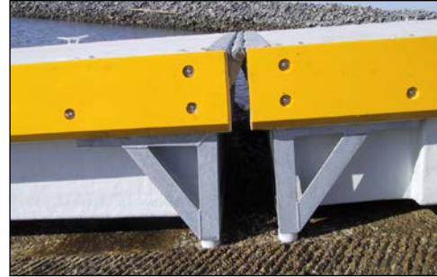
unnneeded downslope support leg(s)
