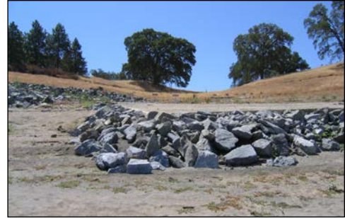
rock rip rap failing at bottom of a lake based boat launching ramp
