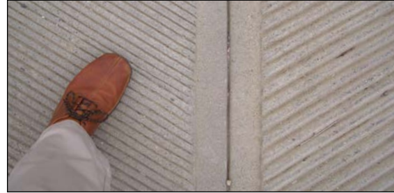
two-lane launching ramp 1 inch V-grooves on right lane 1/2 inch V-grooves on left lane
