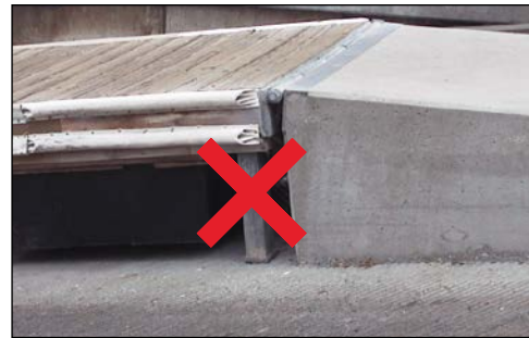
“no-no” float legs next to abutment
